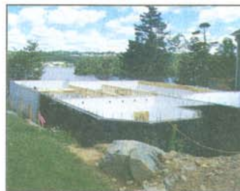
Mike Perrier, Perrier's Concrete Homes, Dartmouth, N.S. is one of few residential contractors in Atlantic Canada who builds exclusively with insulating concrete forms (ICF). Mike and his all-deaf crew have become specialized with the IntegraSpec® ICF wall system over the past five years, raising the building envelope only. This beautiful single-storey home, built last summer, overlooks Lake Banook in Dartmouth.
